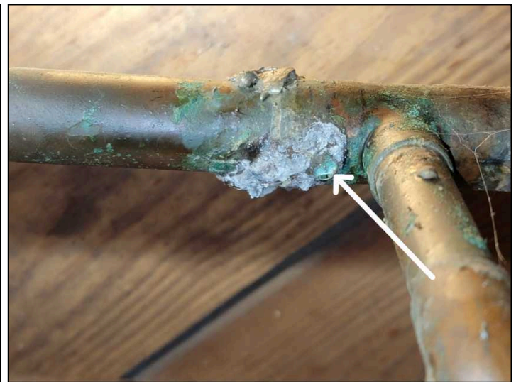
Active Leak observed (Zoomed-In)
