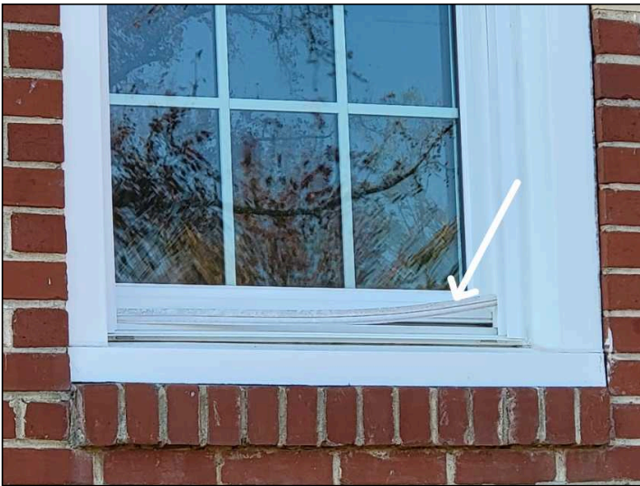
Damaged/Loose Hardware (Right Side)
