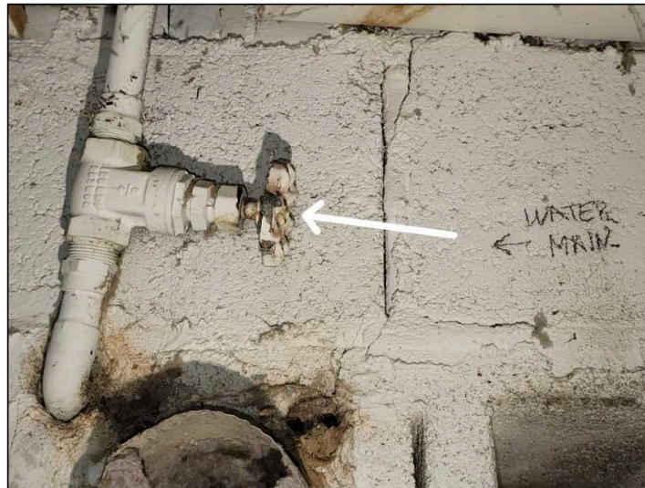
Main Water Shutoff Valve
