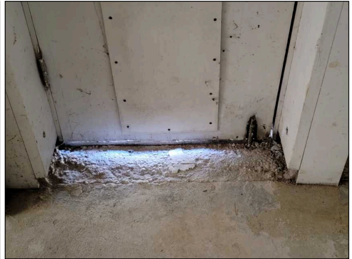
Daylight Visible Under Door (Basement)
