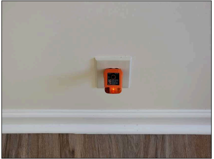
Open Ground (Main Level Front Bedroom) ALL Receptacles
