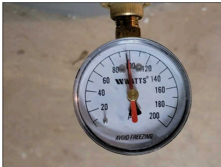
Water Pressure Tested at Approximately (98 PSI)
