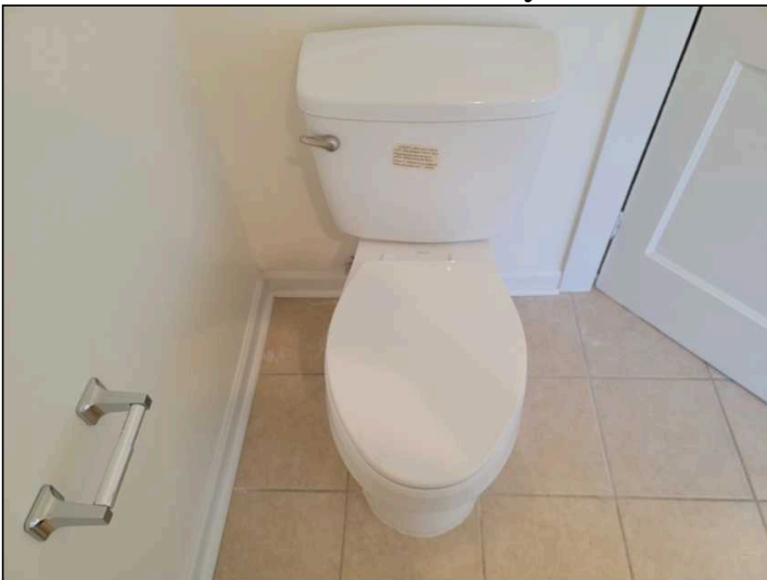
Loose Toilet (Upstairs Guest)
