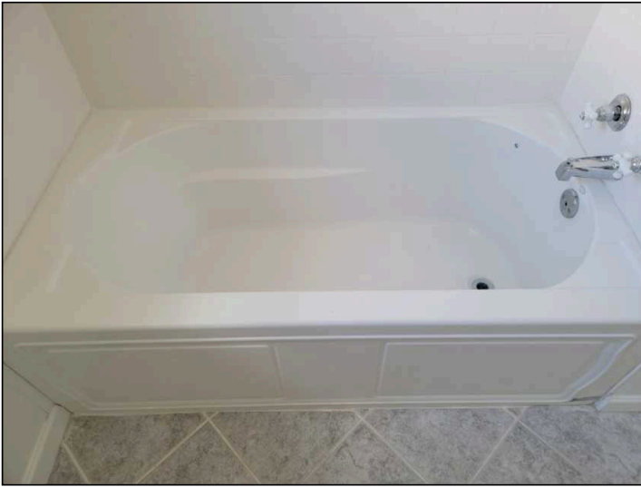
Caulk/Seal All Cracks & Gaps (Guest)
