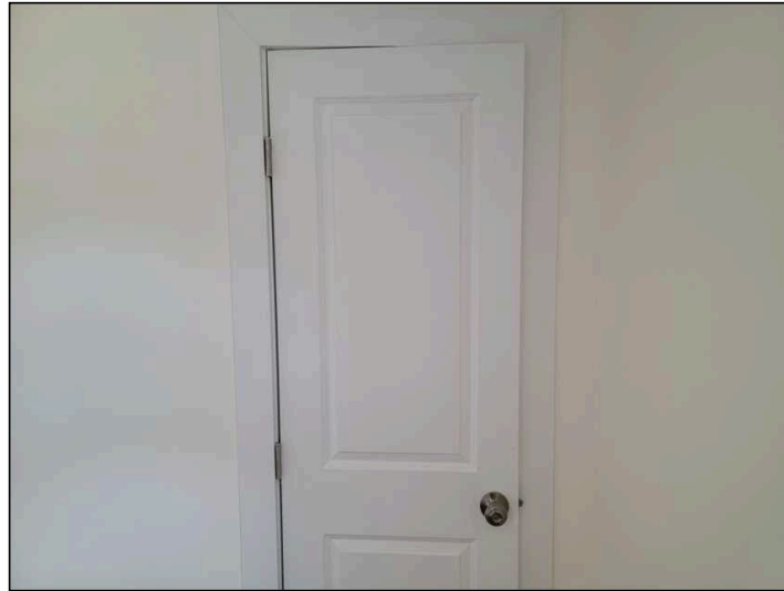
Does Not Close/Latch (Upstairs Right Bedroom Closet)
