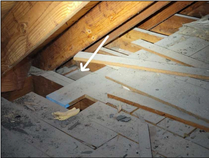
No Insulation over Main Level Front Bedroom
