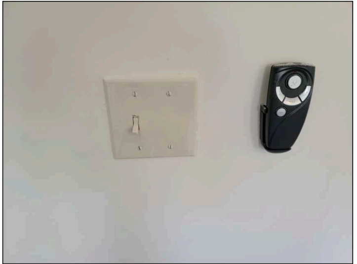
Switch Installed Upside Down (Left Bedroom)
