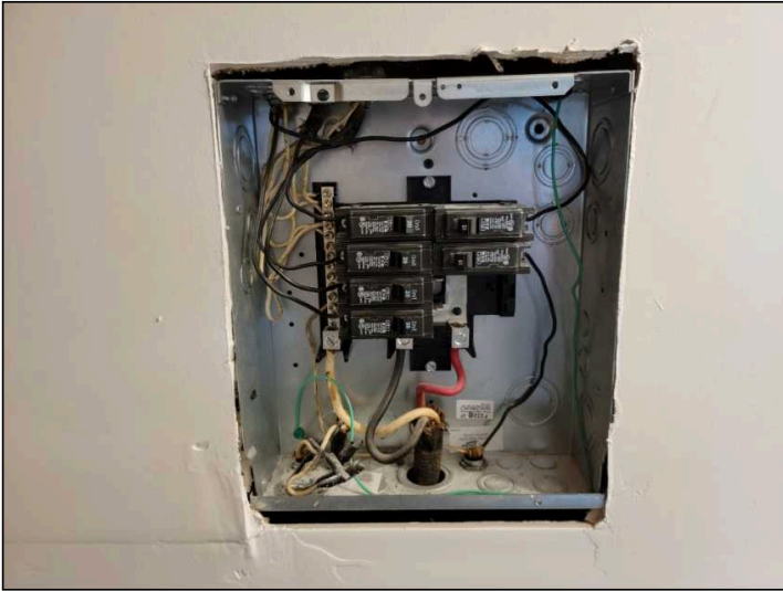
View of 1st Sub Panel
