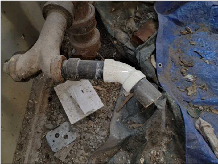
Unprofessional Repairs/Improper Connections
