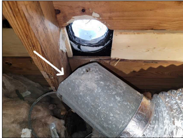
Vent Pipe Not Attached
