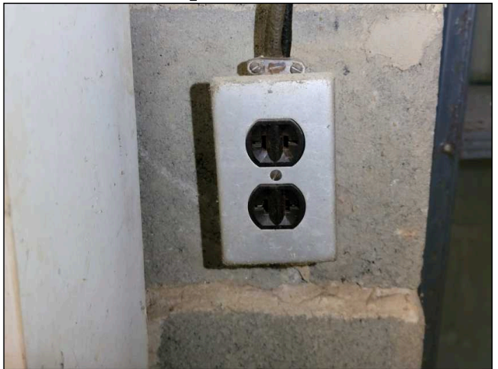
2 Prong Receptacle Noted
