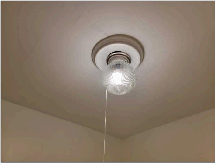
Loose Fixture (Left Bedroom Closet)
