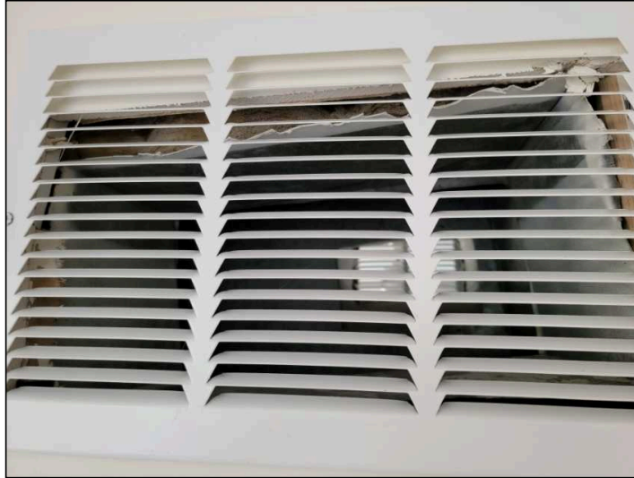
Duct Appears Damaged/Loose
