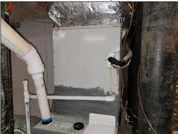
Fan Makes Irregular Noises
