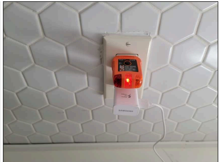
Bad GFCI (Open Ground)
