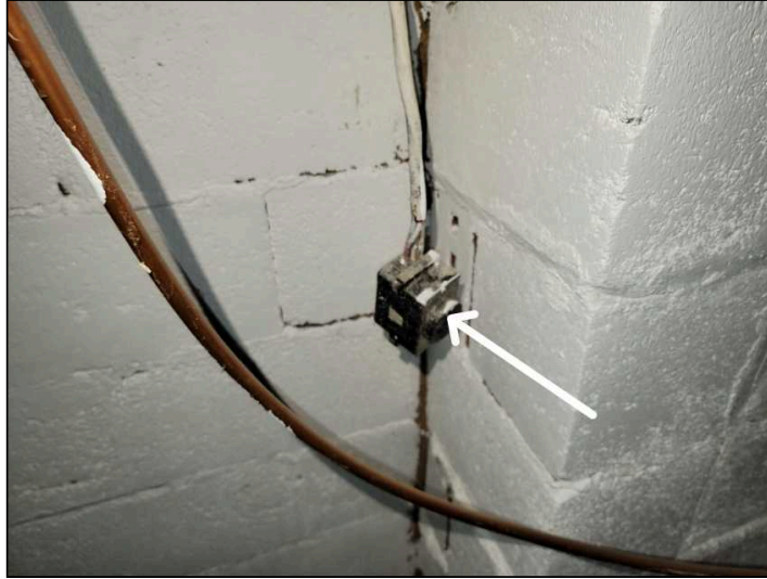
Loose Dryer Receptacle
