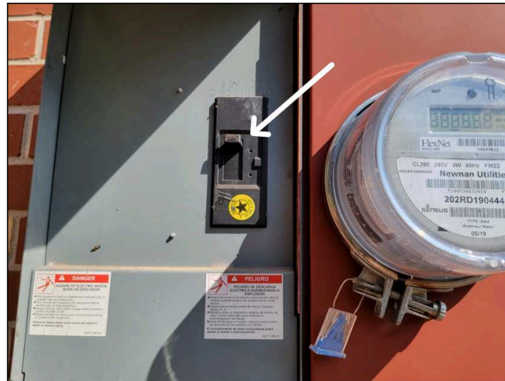
Main Service Breaker
