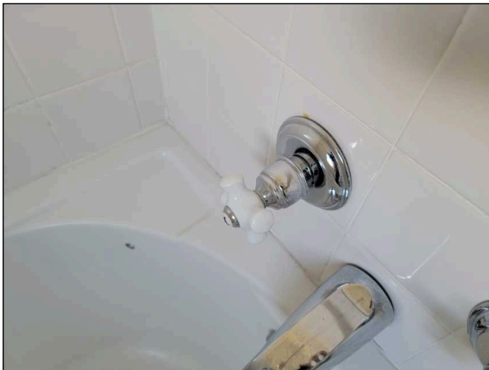
No Hot Water Supply (Guest)
