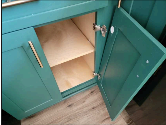
Missing Screws (Both Hinges)
