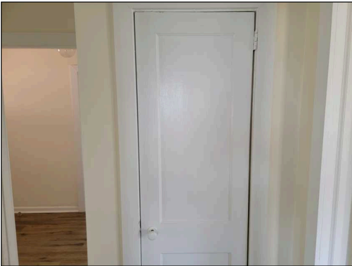
Tight in Jam (Master Bedroom Hallway)
