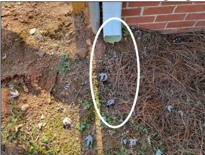
Missing Splash Blocks
