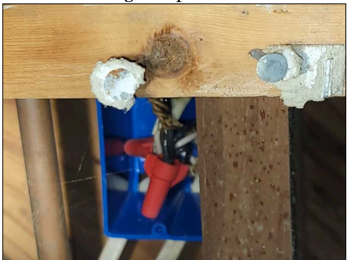
Open Junction Box
