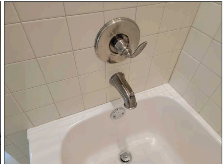
No Hot Water Supply (Upstairs Guest)
