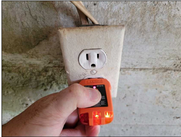
No GFCI Protection
