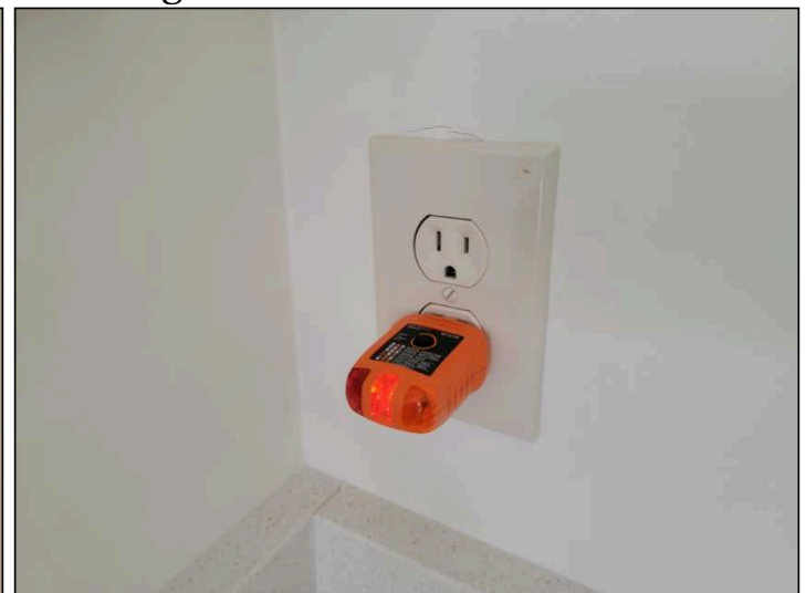
Open Ground & Loose Receptacle (Master)
