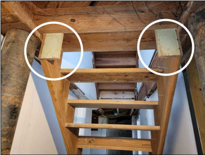
Not Properly Attached/No Supports
