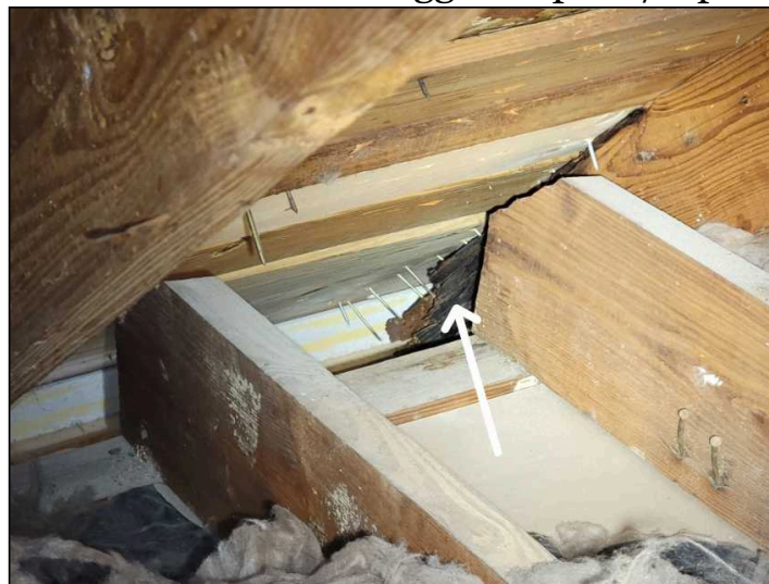
Damaged/Deteriorated Wood (Front Left)
