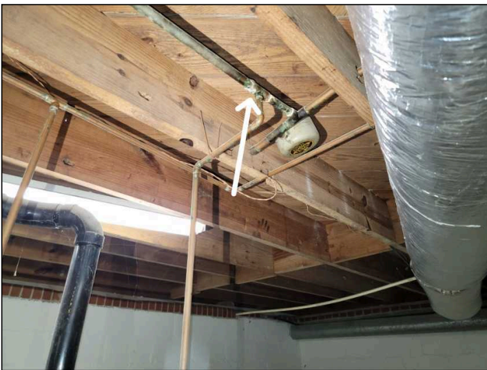
Active Leak Observed (Basement)
