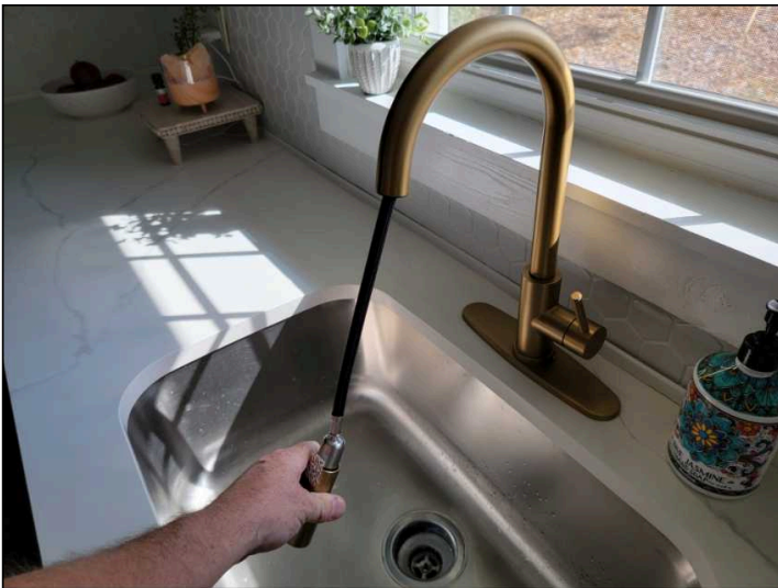
Weight Installed Too High
