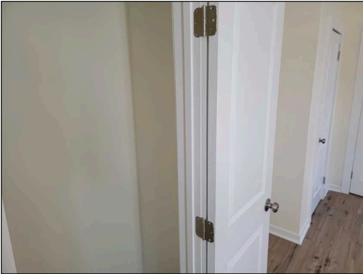
Missing Screws/Hardware (Main Level Front Bedroom Closet)
