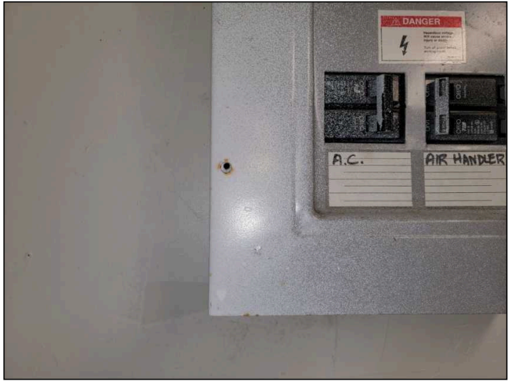
Panel Cover Screw Missing (2nd Sub Panel)
