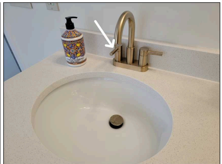
No Hot Water Supply (Master)
