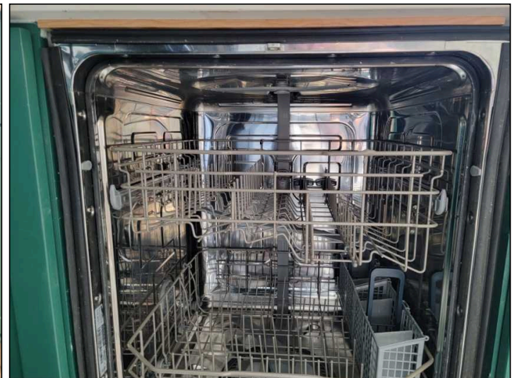
Not Mounted Properly
