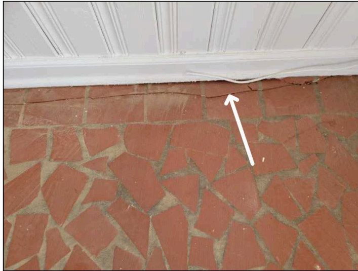
Settlement Crack Noted
