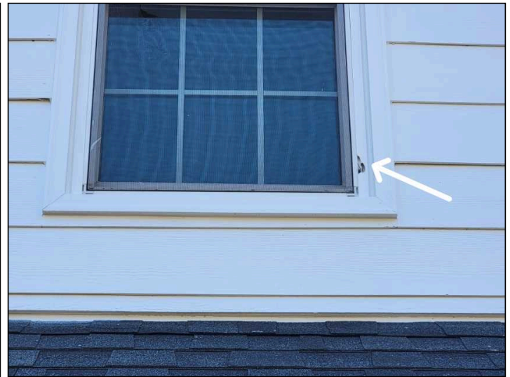
Damaged Frame (Rear)
