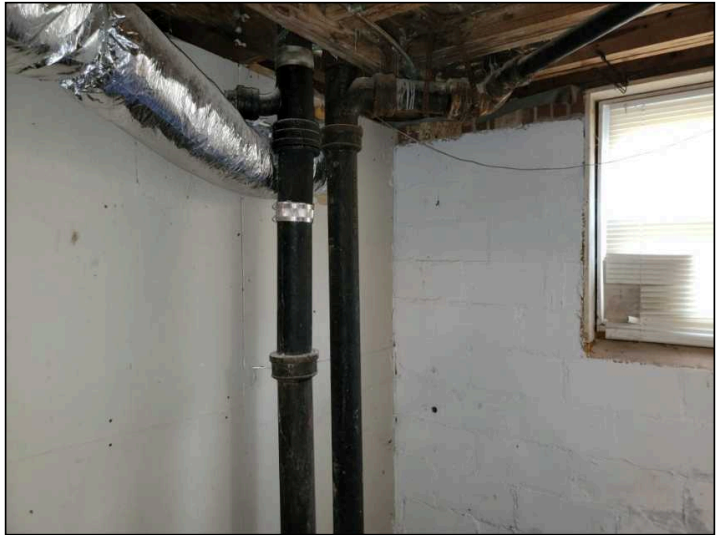
Cast Iron Drain Pipes
