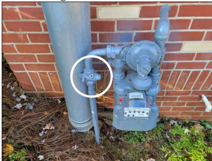
Main Gas Shutoff Valve
