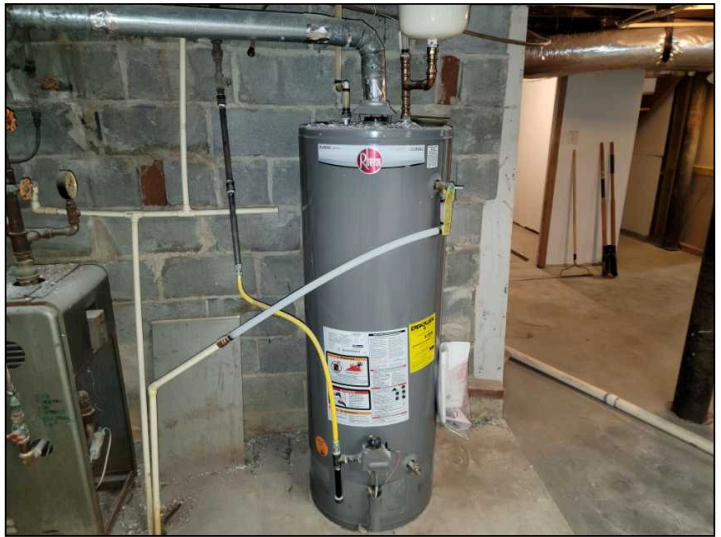
View of Water Heater
